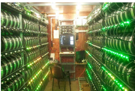
Offshore petroleum exploration hardware Seismic data processing software "On-The-Fly" Optimal work route in exploration acreage
